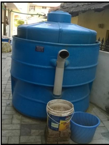
Institute Bio-gas Plant
